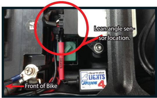
CANopener location on a K1600GT.
